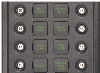
Push Button Circuit Breaker
